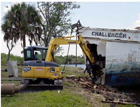
FORT MYERS, Fla. – A bulldozer demolishes the fishing vessel Challenger May 22. The vessel was taken to a Lee County-approved dumpsite for further destruction and disposal where substantial amounts of residual pollutants within the vessel were safely removed. Coast Guard photograph.
